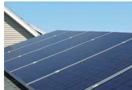
Solar water heating systems are inexpensive to install and may greatly reduce the cost of supplying hot water to a development.
